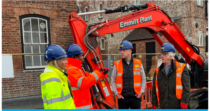
Working with the Environment Agency to get the bridge open before the summer holidays
