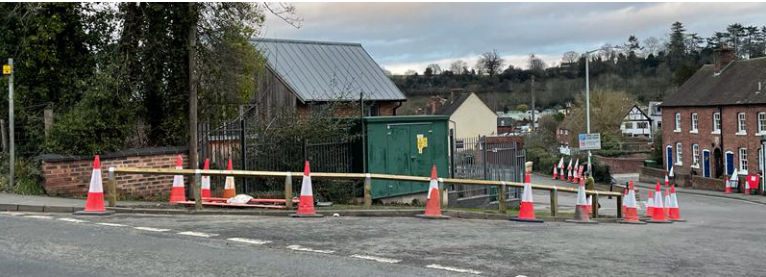
Wooden post and rails have been installed to prevent illegal parking and protect the grass verge
