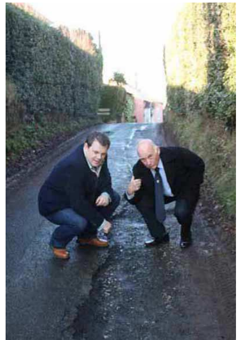
Andrew and Gordon inspecting the bad state of School Lane Trimpley which is in need of resurfacing
